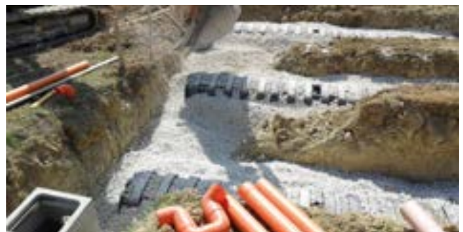
④ COVERING Connect feeding and ventilation pipes. Cover with at least 150-200 mm of gravel 20/40 mm.
