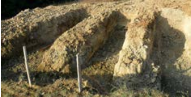
① EXCAVATION Dig a trench at least 900 mm wide at the base.
