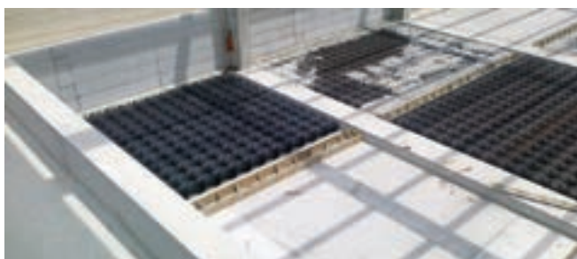
① SLAB ON GRADE Sub-base of gravel and lean concrete, and an HDPE membrane (for compost plants).
