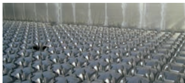
② BIOMODULO INSTALLATION Laying of Biomodulo with caps, Geoblock and Fermagetto. Creation of inspection channels.
