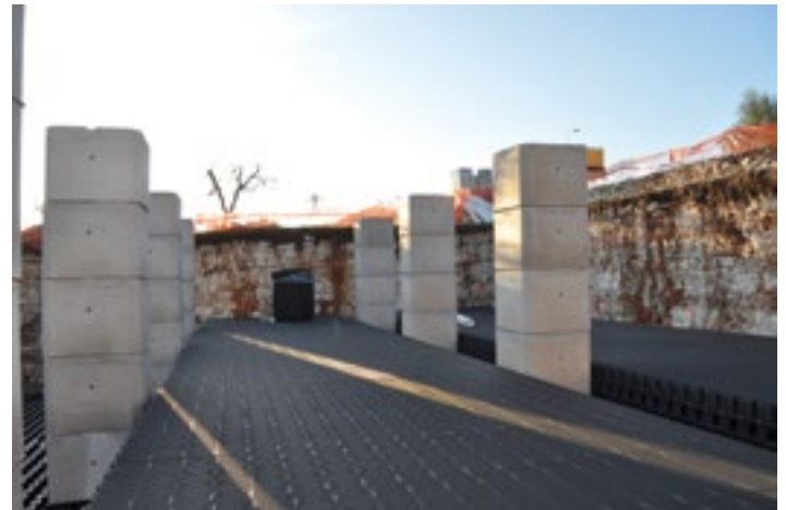
Figure 22 - Manholes for basin cleaning operations
